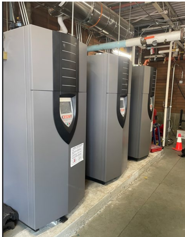
Photo: New Lincoln Square Hydronic Boilers
