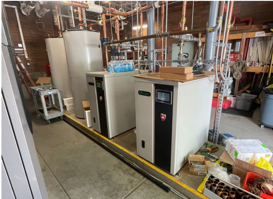
Photo: New Lincoln Square Domestic Boilers
